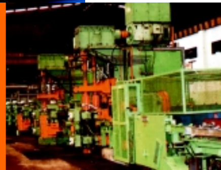
Housingless stands in Amsteel Mills' wire rod mill. Barisan penggulung di kilang rod wayar Amsteel Mills.
